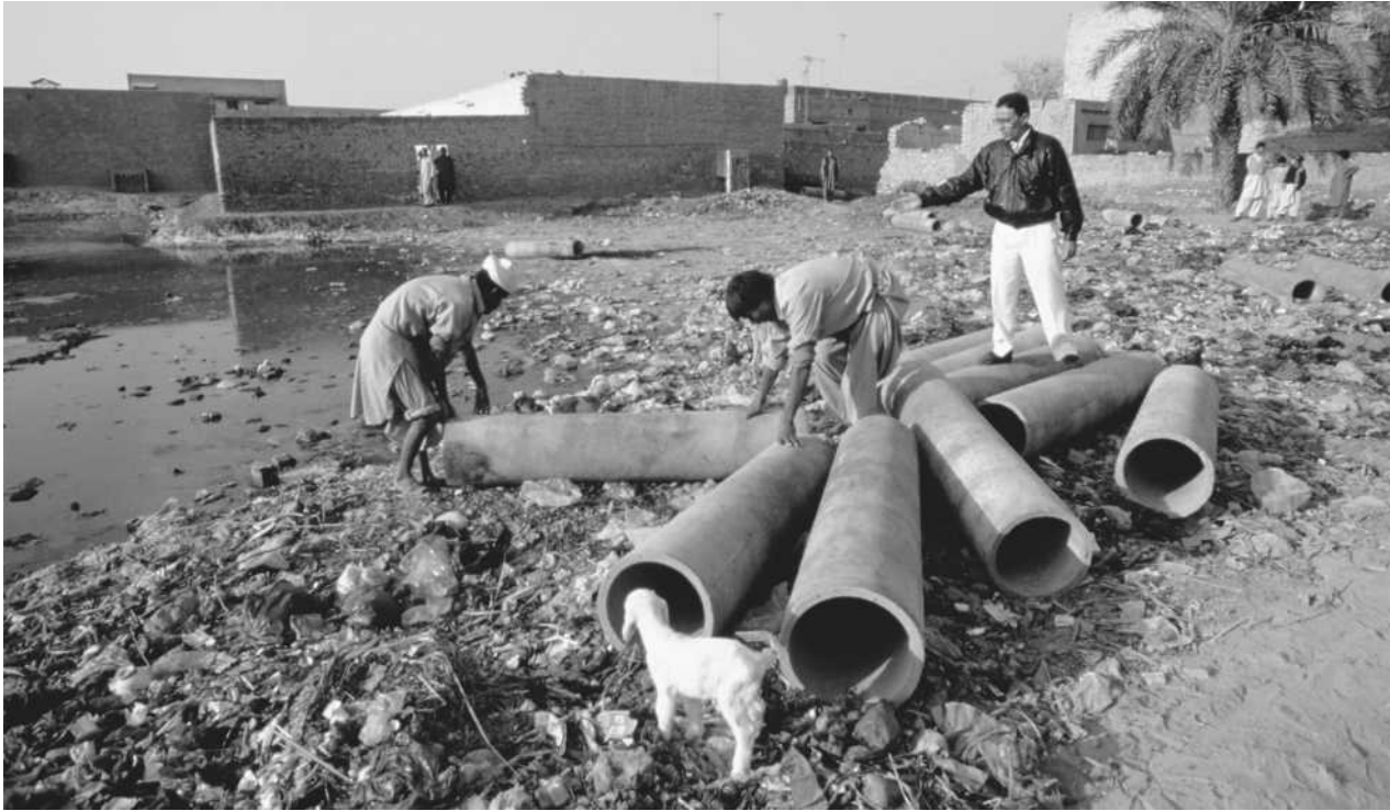
Workers on a community sanitation project examine the pipes for a new sewer in Faisalabad.
